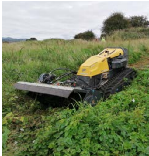
Fence Scape Ltd. used a robotic flail to get hundreds of years of vegetation growth under control.
