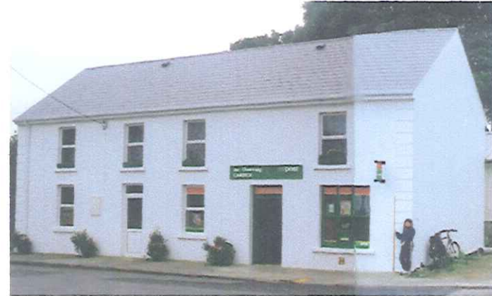
Illust. 8 - In the nicely refurbished Oifig an Phoist at An Charraig, The chimneys were covered over by the roofer. Following the 'Final Public Participatoin Consultative Meeting', the owners have said that the chimneys are still beneath the roofing slates and they will rebuild them again soon
