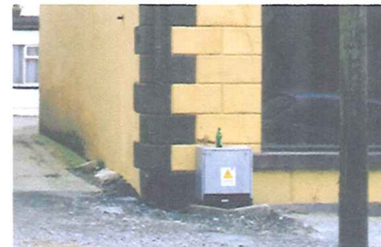
Illust. 18 - The obtrusive ESB meter boxes
